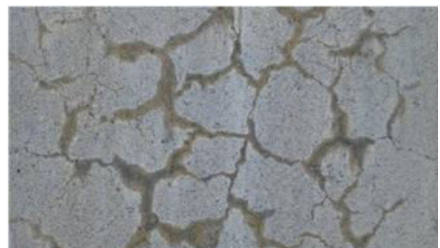
Fig. 4. The pattern cracking effect due to alkali silica reaction.
