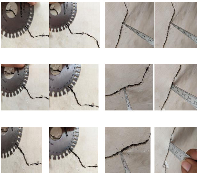
Fig. 5. Case study 3 displaying the measurement of the cracks in a structural component.
