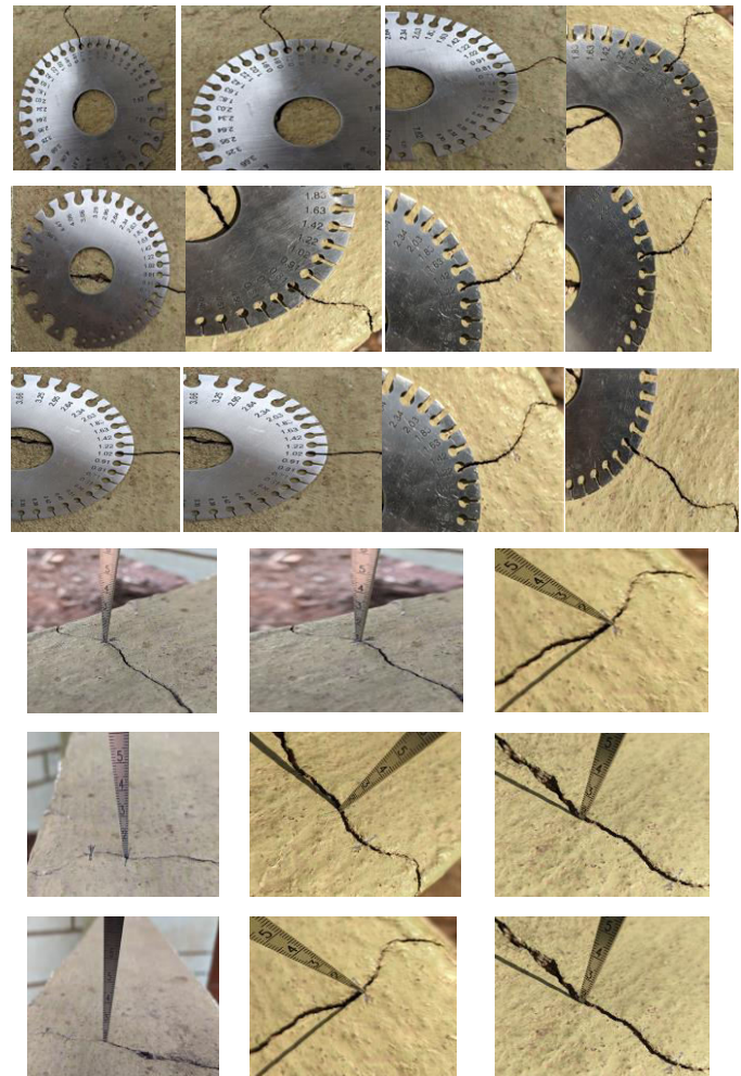
Fig. 1. Case study 1 displaying the measurement of the cracks in a structural component.
