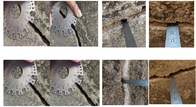
Fig. 3. Case study 2 displaying the measurement of the cracks in a structural component.
