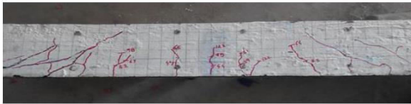
Figure 11. Crack Pattern for Control Beam
