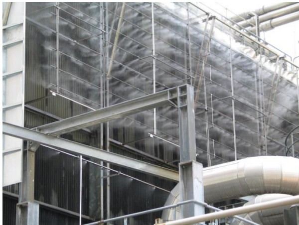
Picture:2: Adiabatic cooling in action
