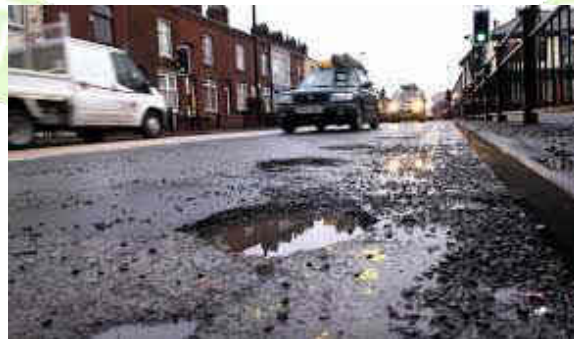
Figure 1: potholes on the road
