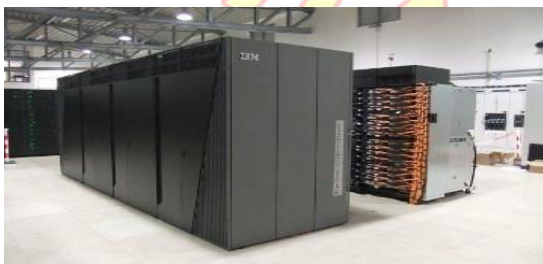
FIGURE7: JUQUEEN supercomputer in Germany
